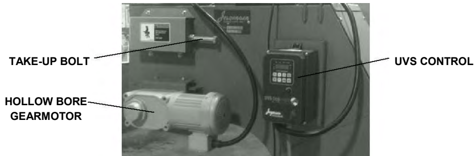
Figure 5: Direct drive side of conveyor
