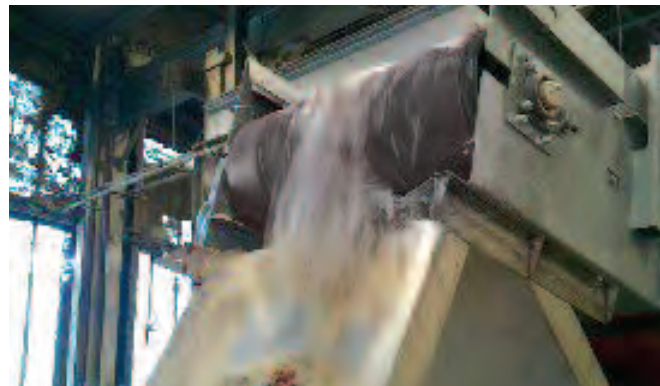
Head Pulley working in an industrial application
